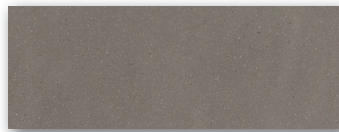
WEATHERED CONCRETE (WX PK: 3)
